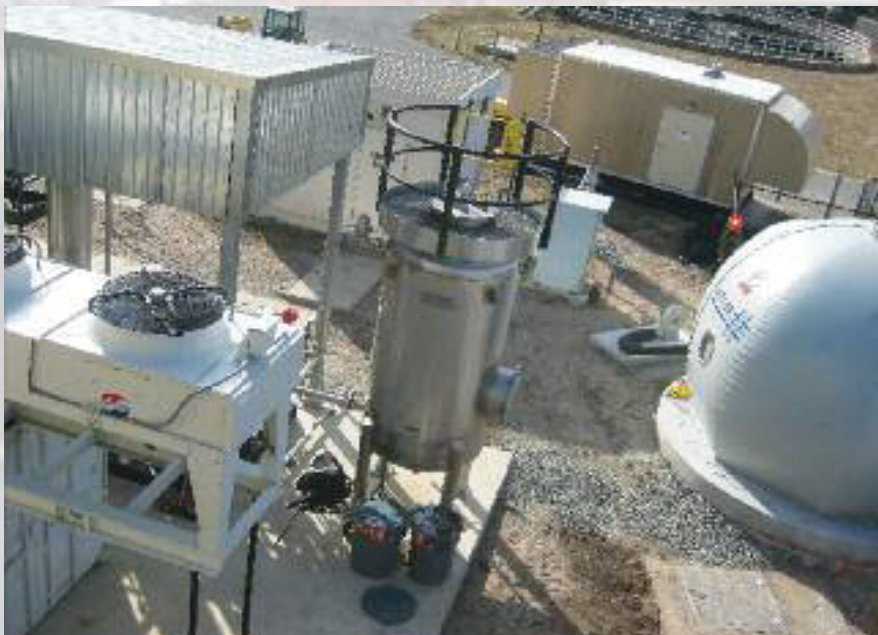
Progress continues on the installation and integration of various components of the anaerobic digestion system at the Ridgewood, NJ wastewater treatment plant.
