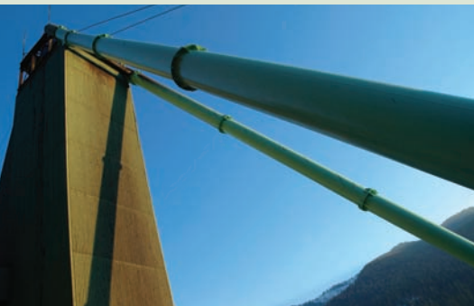
The headframe of the 67-year-old Lucky Friday mine rises high in the mountains of northern Idaho. With decades of resources identified, the deposit appears to grow richer as the mine goes deeper.
